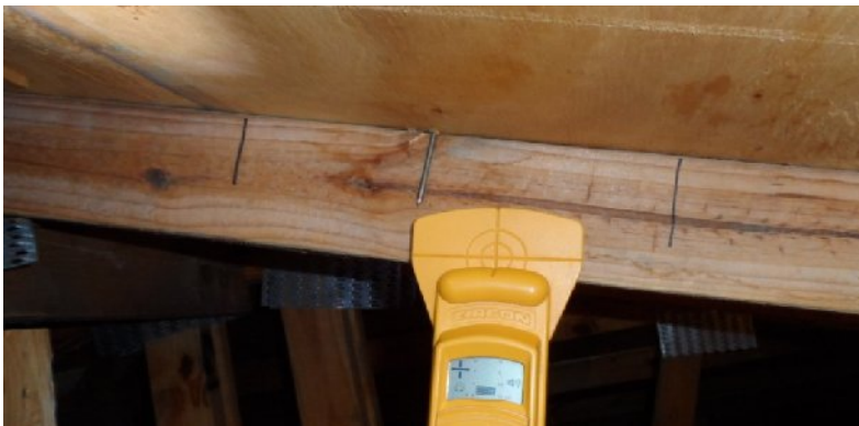
Nail location verified
