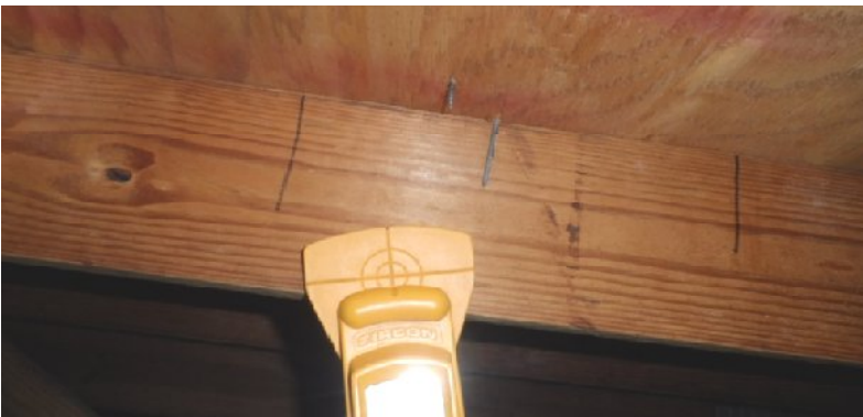
Nail location verified
