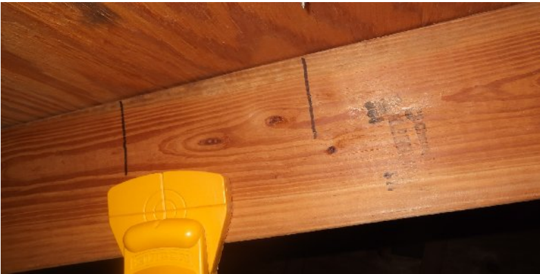
Nail location verified
